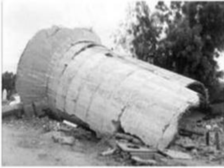
Fig. 1 Collapse of water tank in Bhuj
