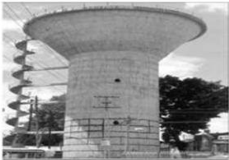
Fig. 2 Flexure cracks in staging
