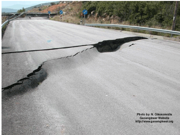
Fig.1.1 - Failure of pavement due to expansive soil
