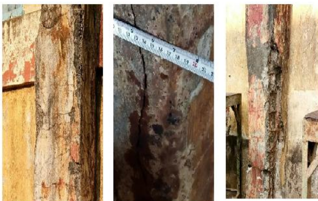
Hairline Cracks on column
