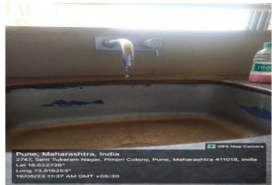
Fig 5: Improper closing of valve
