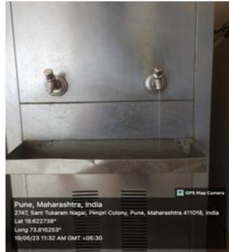
Fig6: Leakage in taps
