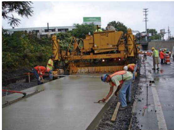
Figure 8 Plastic concrete extruded to correct grade and the cross slope behind the slip-form paver.
