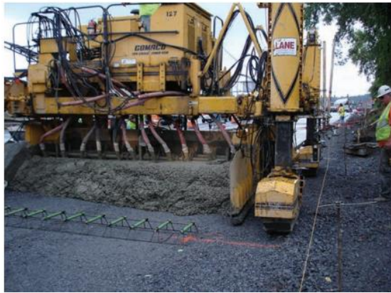
Figure 7. String line controlled slip-form paver approaching dowel basket (note vibrators for consolidation).
