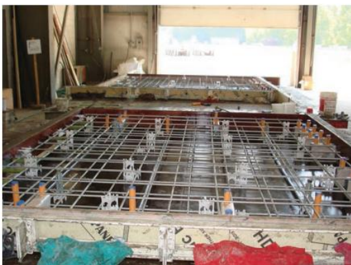
Figure 4 Two layers of reinforcing steel in each direction in a JPrCP fabrication
