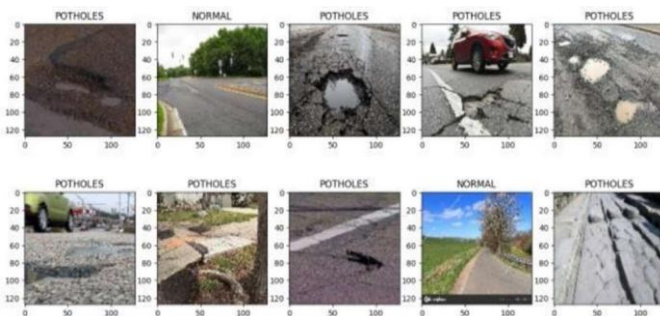
Fig 1. Trained Images of Potholes
