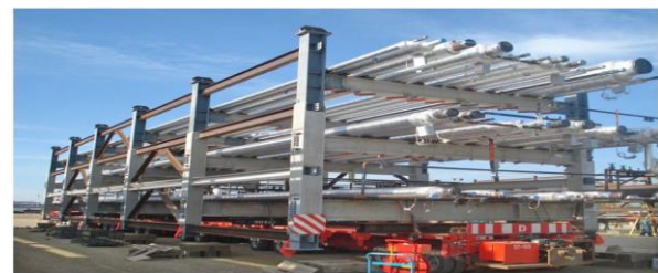
Fig. 3.8. Industrial module construction prefabrication and preassembly facility (photo courtesy of U. Hermann, PCL)
