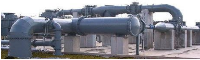
Figure 1. Duplex stainless steel used in Desalination Plant
