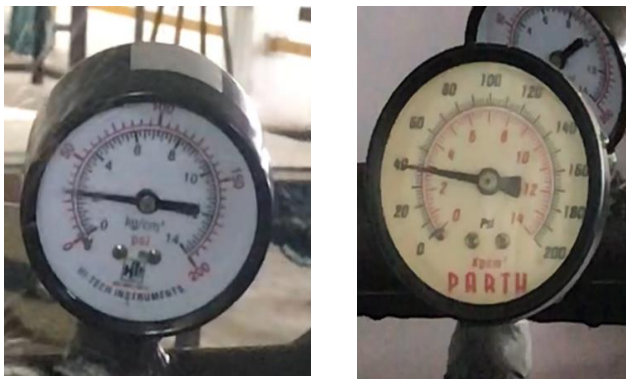
Fig. 3. Readings Shown by Pressure Gauge.
