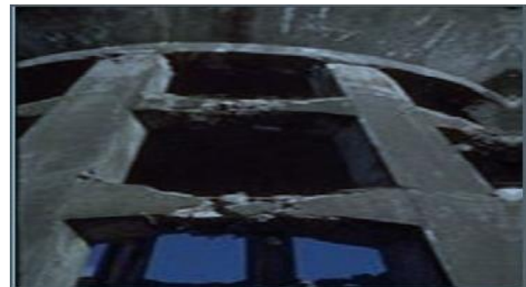
Fig. 1 : Bending Shear Failure in beam
