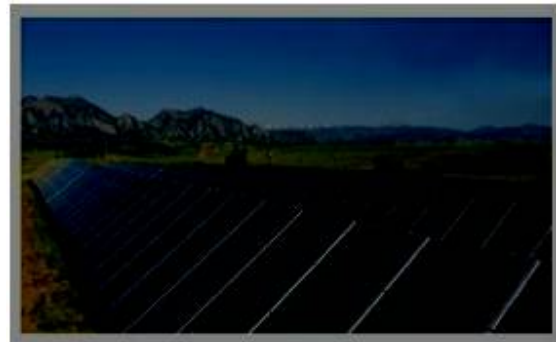
Figure 2.2.I Solar arrays in field [10]
