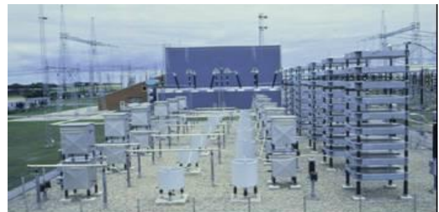
Figure 1.6: HVDC Converter Station HVDC
