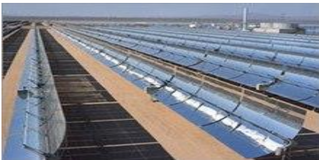
Array of parabolic troughs
