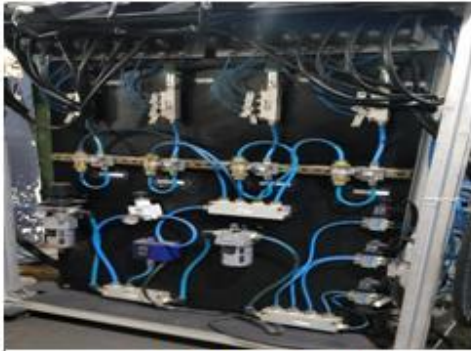
Fig.32 Pneumatic Circuit board
