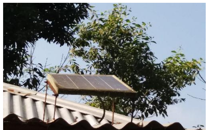
Figure 3: Pico-Solar Panel Set Up on the House Roof
