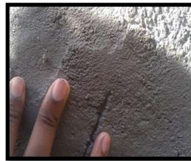
Figure 4.4.2- At 0.3% Plaster Patch With Cracks
