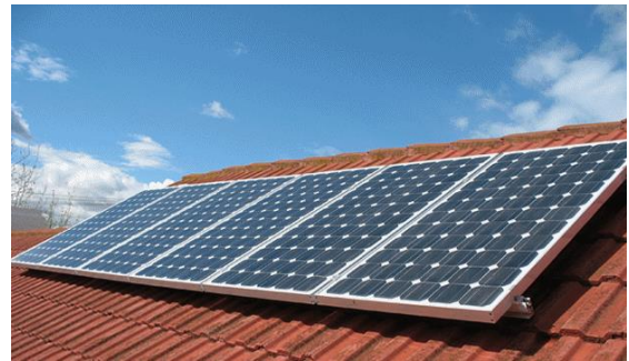
Fig. Solar Panel
