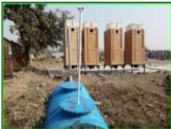
Fig 17: Bio Digester at Depot
