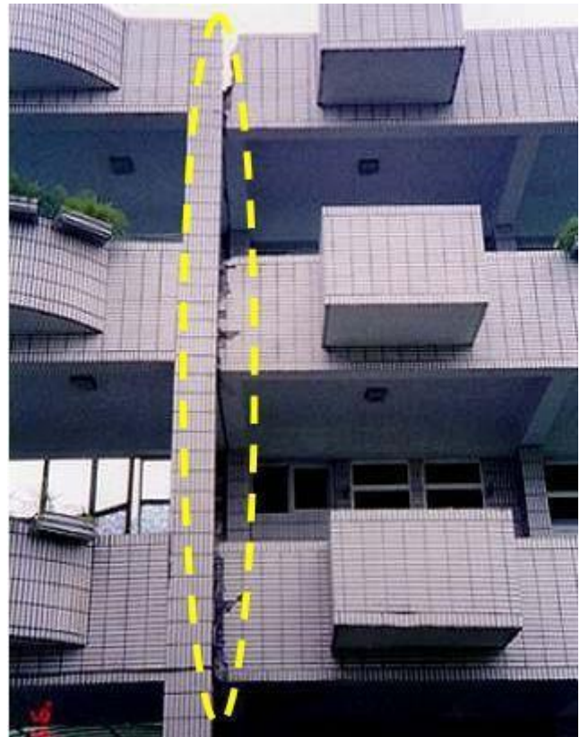
Fig-1 :Pounding of Adjacent Buildings
