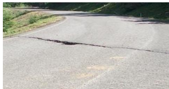
Fig 2.1: Sub-grade failure crack
