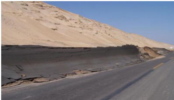
Fig2.2: Failure Of Slopes
