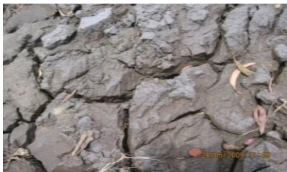
Fig 2.3 Cracks in Marine Clay Deposits
