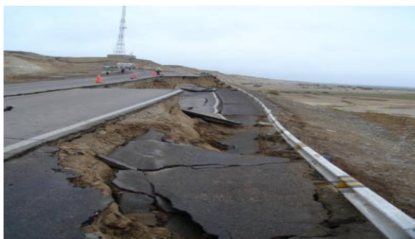
Fig 2.4: Failure of Pavement
