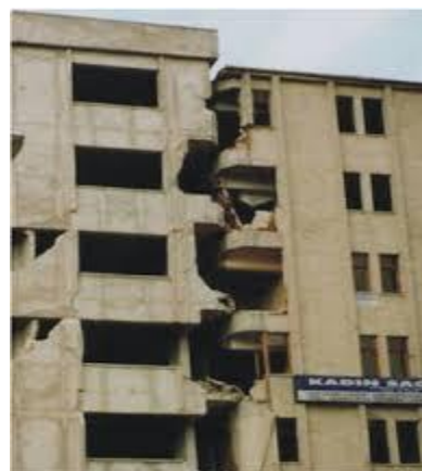
Fig-2 :Pounding of Adjacent Buildings
