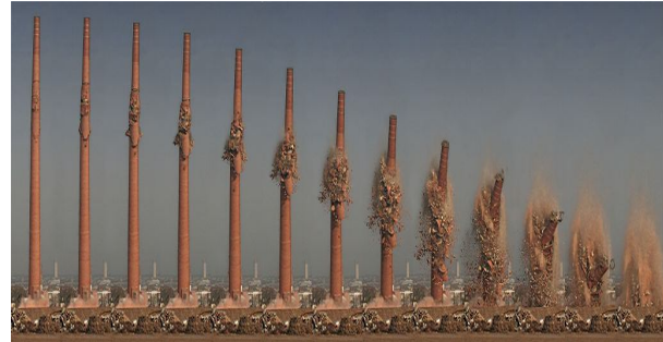
Fig 3-Demolition of a chimney at the former brewery "Henninger" in Frankfurt am Main, Germany, on 2 December 2006
