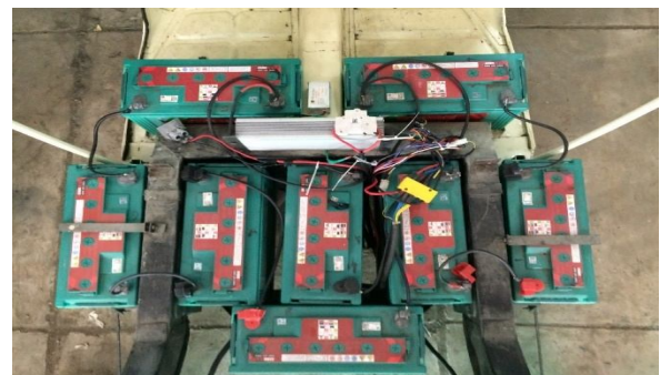
Fig.1 Lead Acid Batteries
