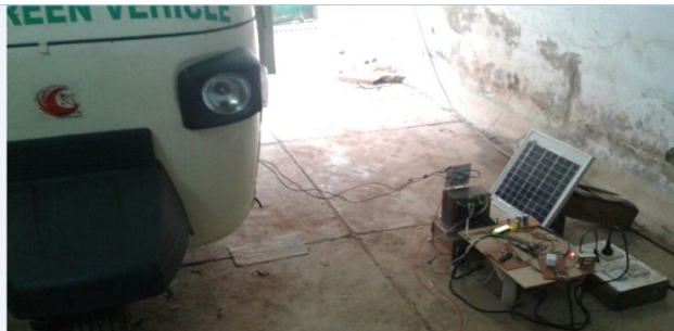
Fig.7 Original Picture of Complete Assembly of Charging Station.
