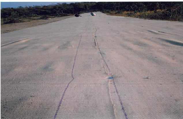
Fig. 5.3 Overlapping and Nailing of Jute Geotextile on the prepared subgrade on both side
