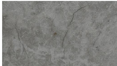
Fig.8 Plastic shrinkage crack in Plain concrete specimen
