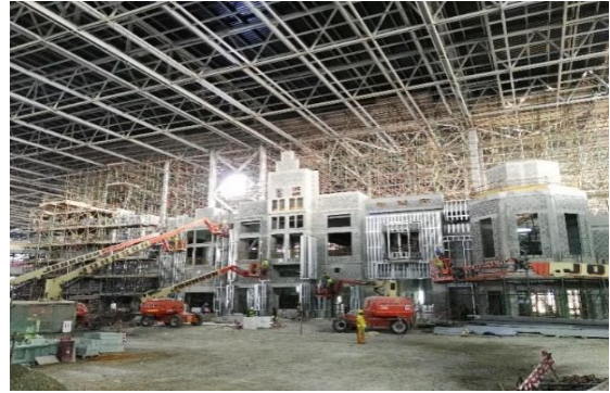
Figure 2(b): WARNER BROS. PLAZA – Structure Works in Progress Theme Façade Handed Over to ASPE
