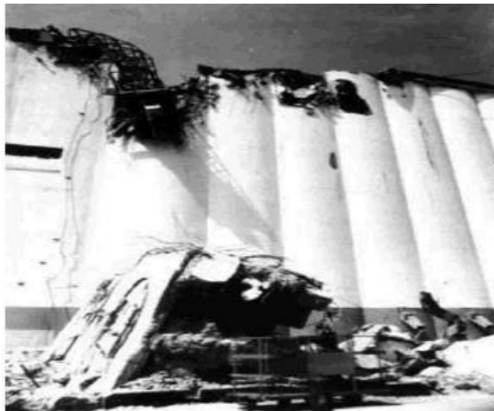
Fig. 1 Partial collapse of grain silo during 1974 Lima, Peru earthquake
