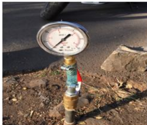
Fig: Meter gauge showing zero pressure
