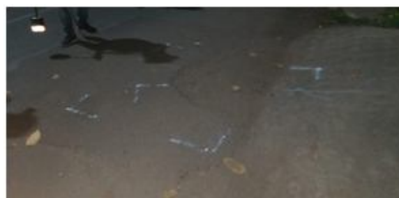
Fig: Identification of point showing Leakage
