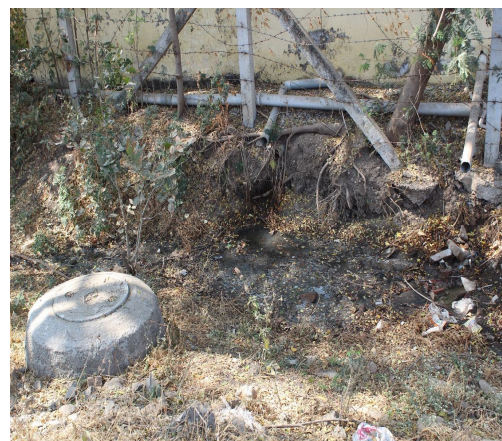
Fig. 8 water logged area
