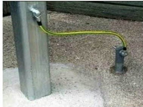
Fig- Pipe Earthing
