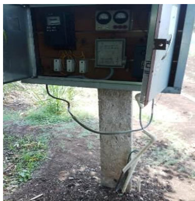
Fig- Proper earthed motor pump
