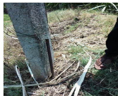
Fig- Improper Earthing
