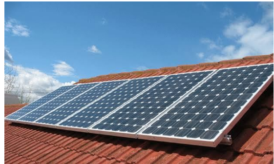
Fig. no. 3 Solar Panel
