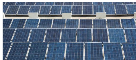
Fig. 1. Solar power panels on the rooftop
