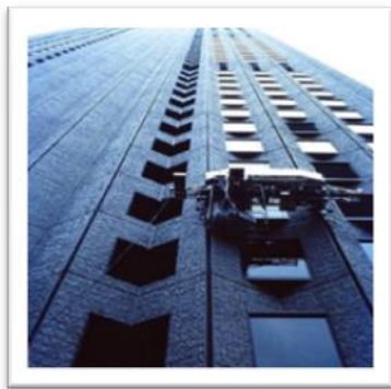
Fig. 2 Single-task construction robot (STCR) applied by the company Taisei to automatically coat and paint the facade of a high-rise building.
