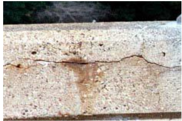
Figure 5. Corrosion of steel reinforcement due to atmospheric pollution
