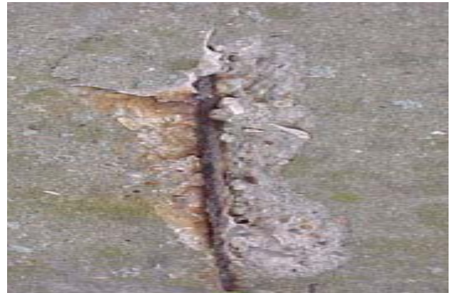
Figure.3 Corrosion of Rebar
