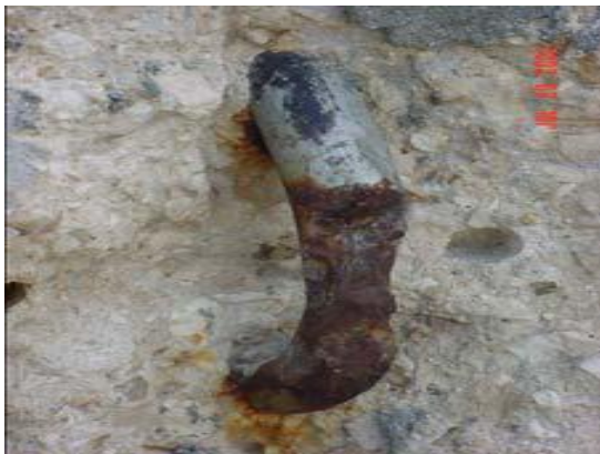
Figure.2 Pits Effect on Steel Reinforcement
