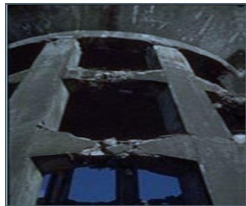
Fig. 1.1: Bending Shear Failure in beam
