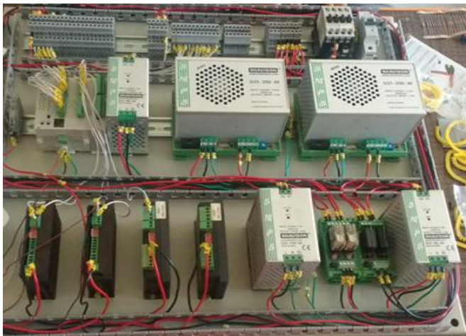
Figure 9. Control Panel Of Developed System
