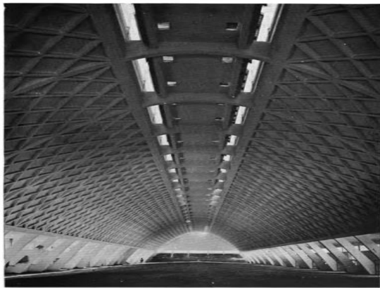
Fig1.3: Ferrocement-roofed warehouse in Tortona, Italy, for storing salt, designed and built by Nervi, 1950-51.
