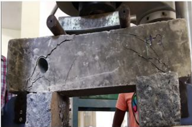
Figure 6: Crack Pattern observed in H2 Specimen
