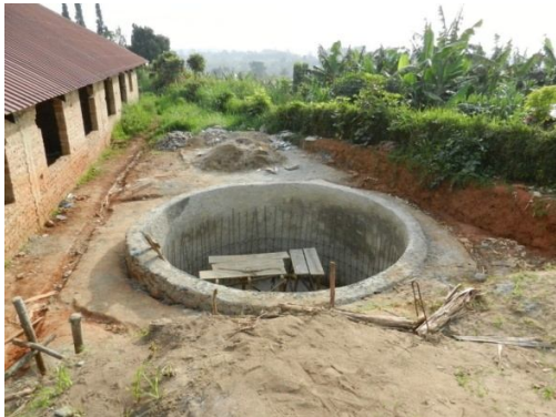
Fig.1.1.2 Underground Water Tank
