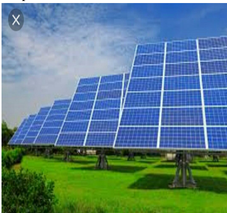
Figure 2. Photo voltaic system
