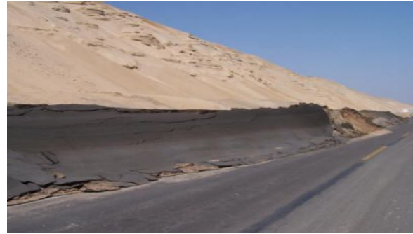
Fig2.1: Failure Of Slopes
