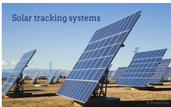
Fig. 1 solar tracking system
