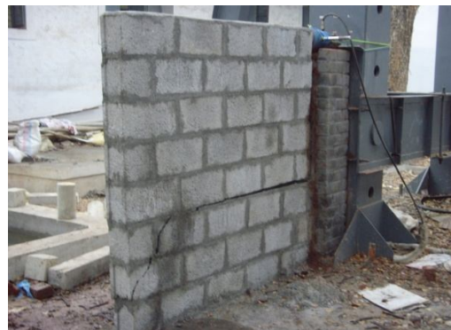
Fig 6.6 Crack occurred in hollow block masonry with fibre reinforcement
