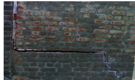
Fig 6.5 Crack occurred in brick conventional masonry
