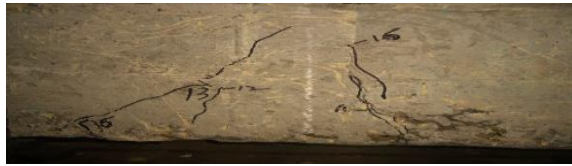
Appearance of beam after testing
