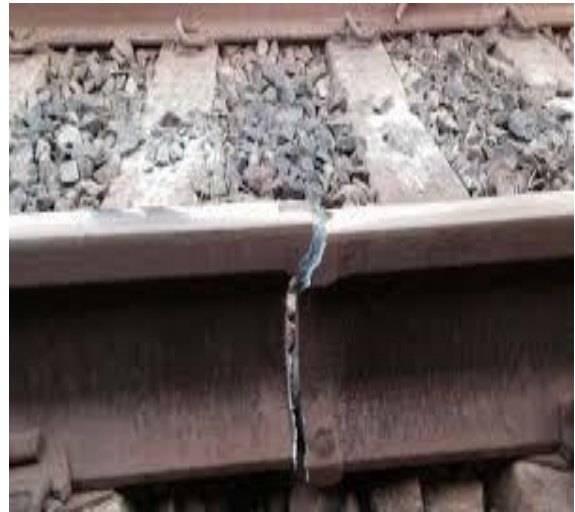
Fig 1: Crack on track
