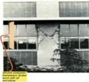
X-shaped cracking damage due to short column
