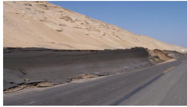
Fig2.2: Failure Of Slopes
