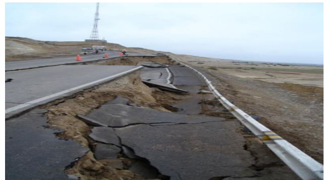
Fig 2.4: Failure of Pavement
