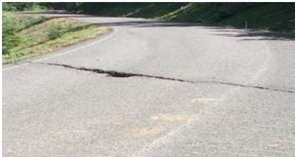
Fig 2.1: Sub-grade failure crack
