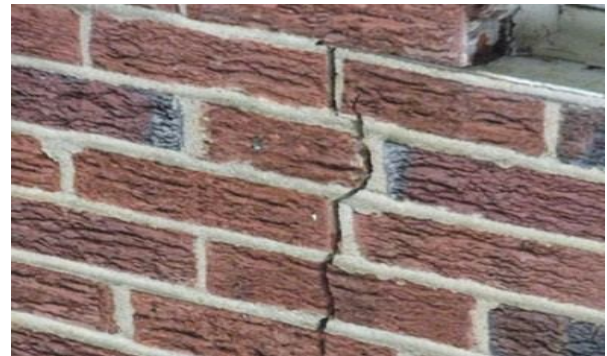
Plate 2.4 Settlement Cracks in SuperStructure Lay on Marine Clay Foundation Bed
