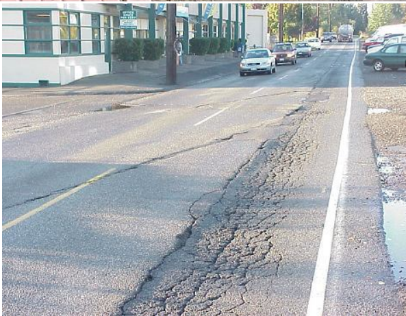
Plate 2.2 Rutting on Pavement of Subgrade
