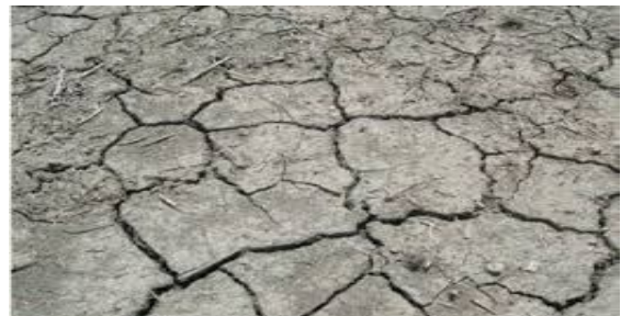
Plate 2.3 Marine Clay Showing Cracks
