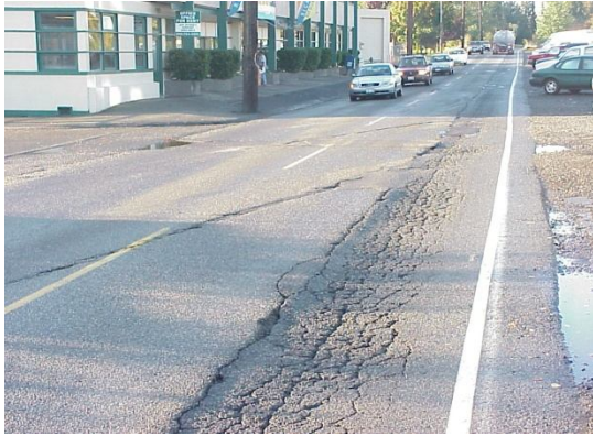
Plate 2.5 Pavement cracks Due to Sub grade Failure
