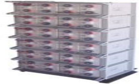
Fig.5) Example of Battery Bank
