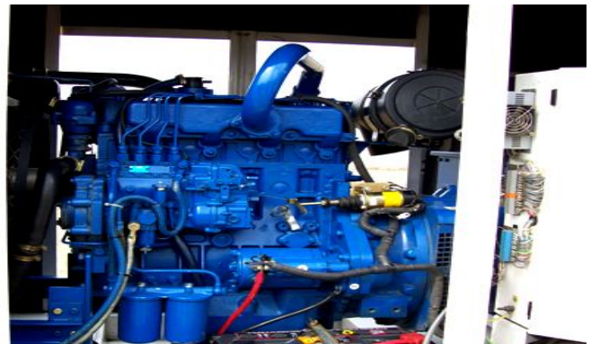
Fig.2) Example of Diesel Generator
